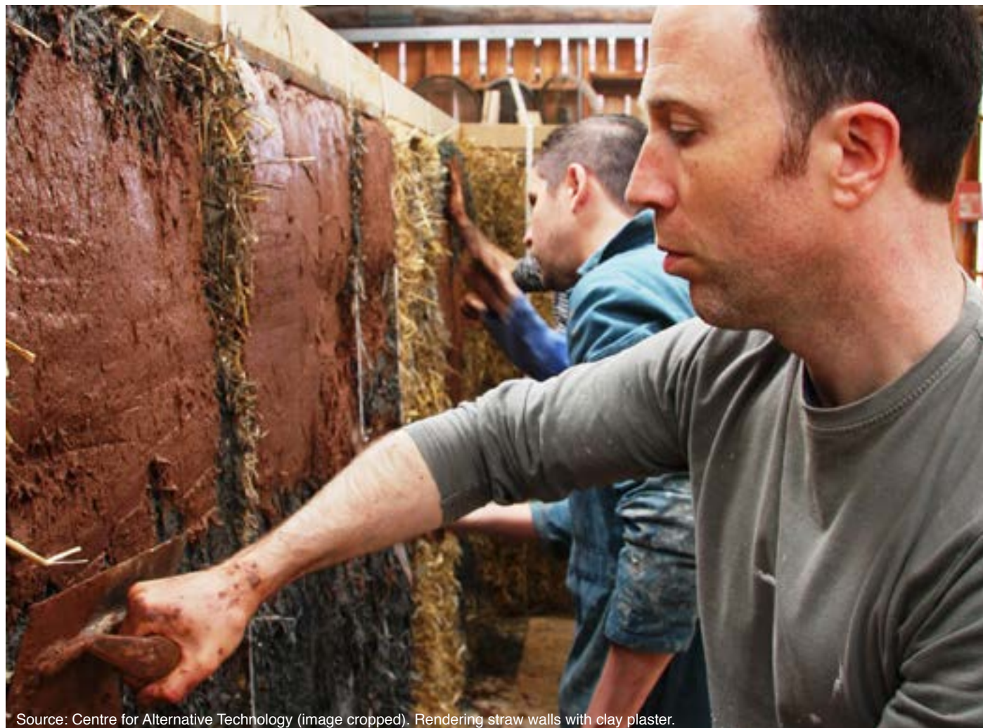
Source: Centre for Alternative Technology (image cropped). Rendering straw walls with clay plaster.
