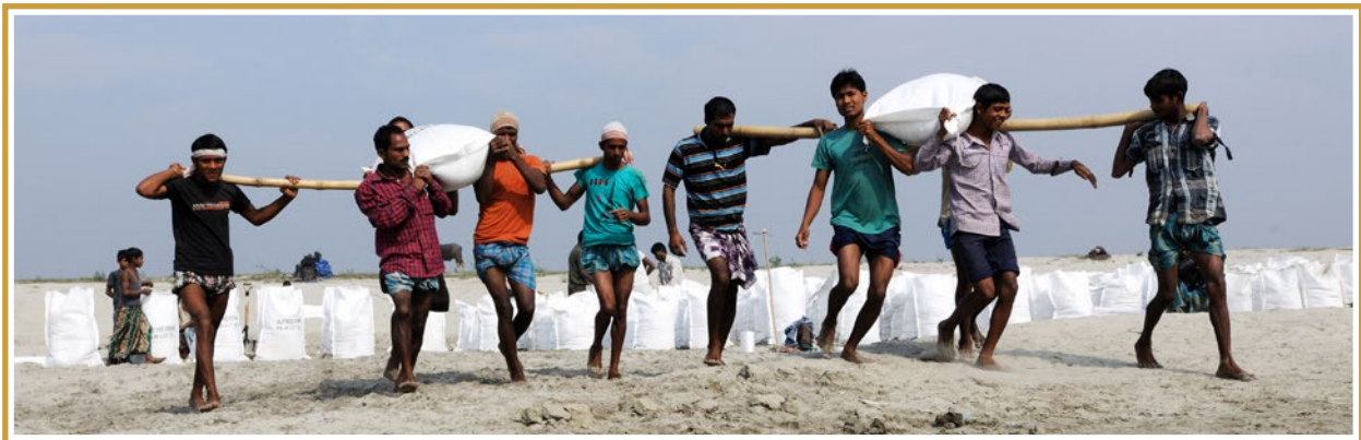
Workers carrying sand filled geo bags to be pitched on the banks of the river Brahmaputra in Gumi village, Guwahati as part of the Assam Integrated Flood and Riverbank Erosion Risk Management Investment Program. Photo: Rakesh Sahai for ADB
